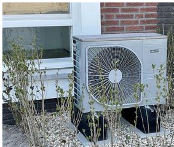
The outdoor unit of a heat pump system.
